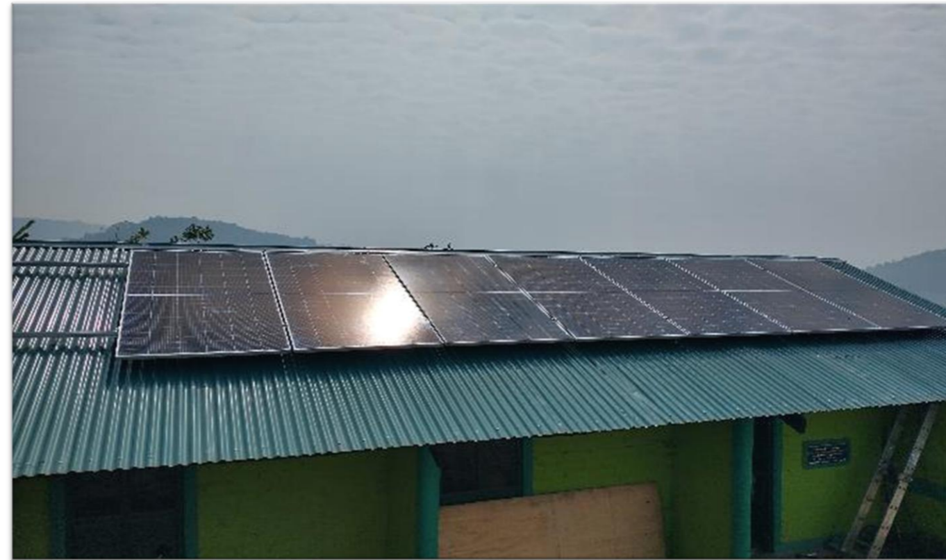
7 kWp Solar and 15 kWh battery back-up in off-grid mode at Amasiko Green Schools, Kabaale.
