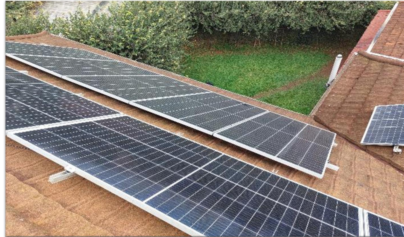
35 kWp solar system with grid connection at Yujo Izakaya Restaurant Kampala.
