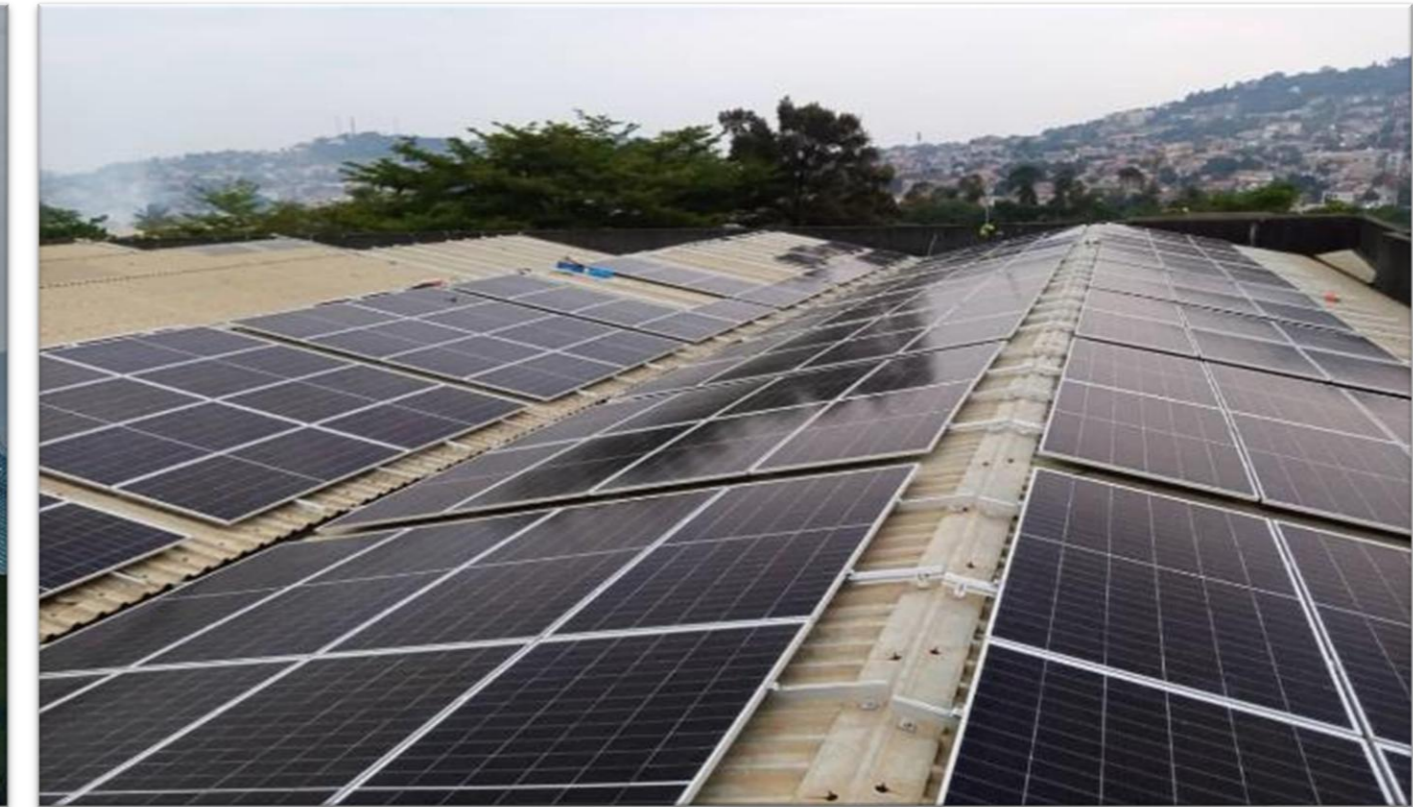
130 kWp Solar PV solution at Internation University o East Africa, Kansanga.
