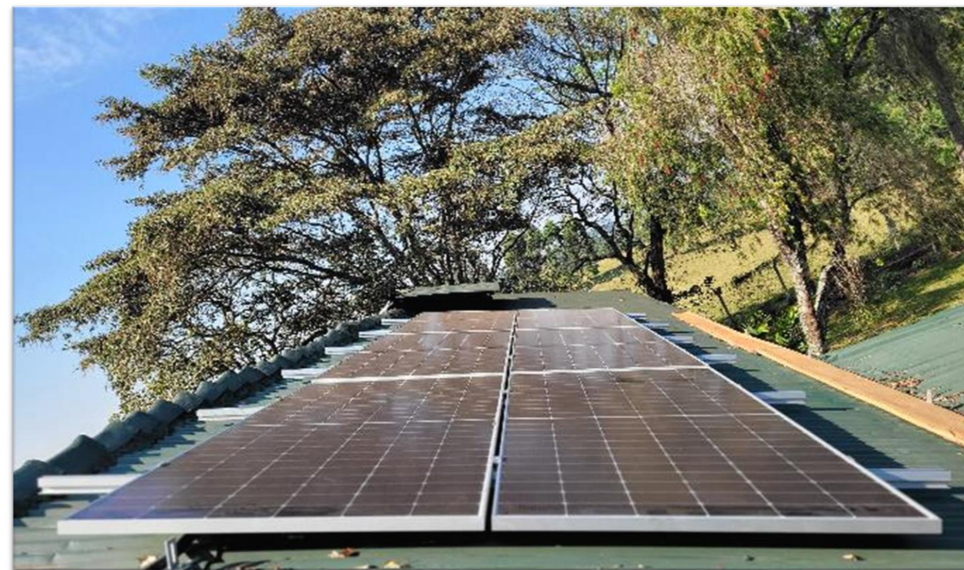
5kWp solar PV and 10kWh battery at Rukararwe Eco Travel Cottages , Bushenyi.
