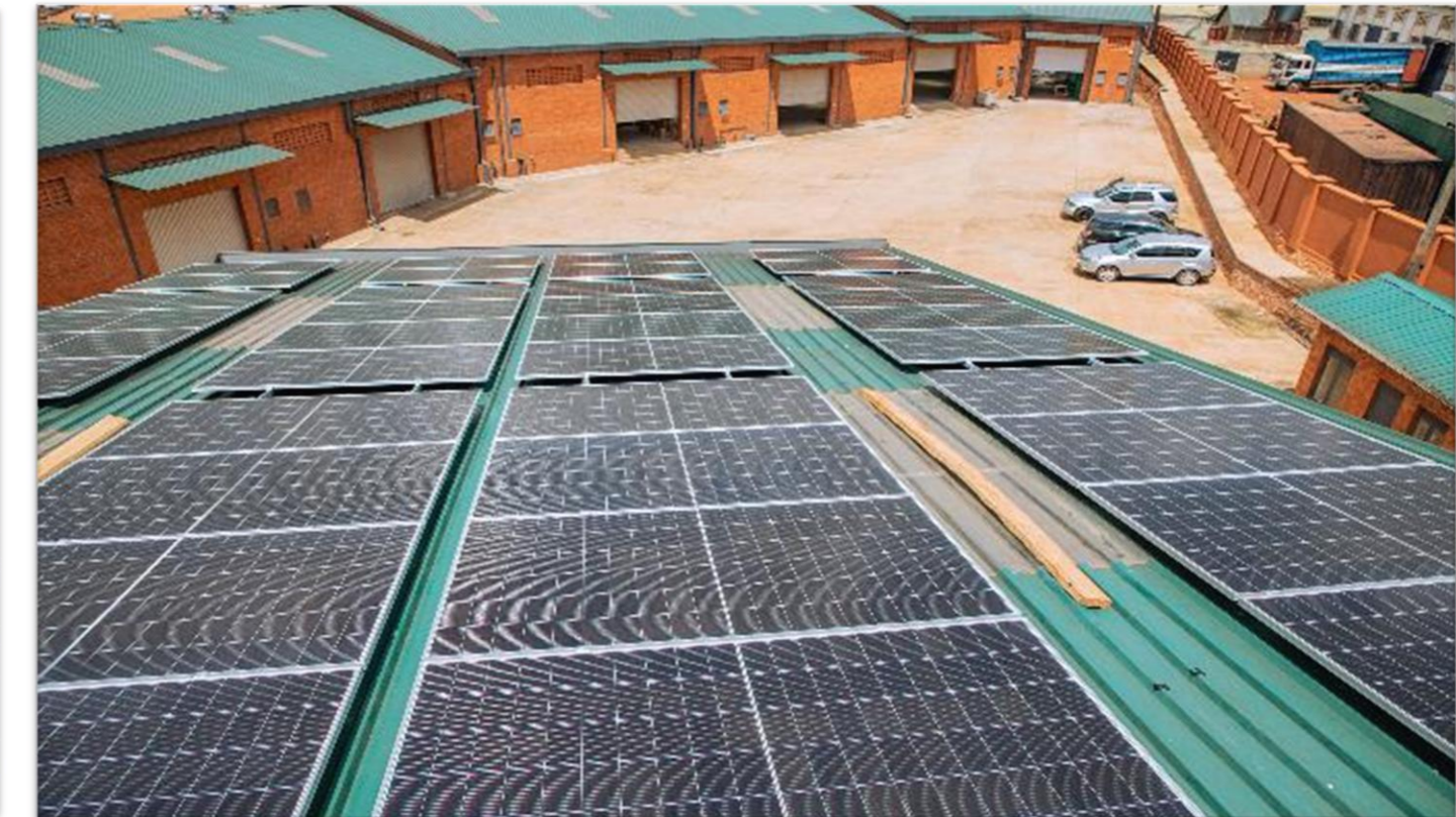
150 kWp solar panels Grid + Generator integration Ranchers Finest Factory , Bwaise.
