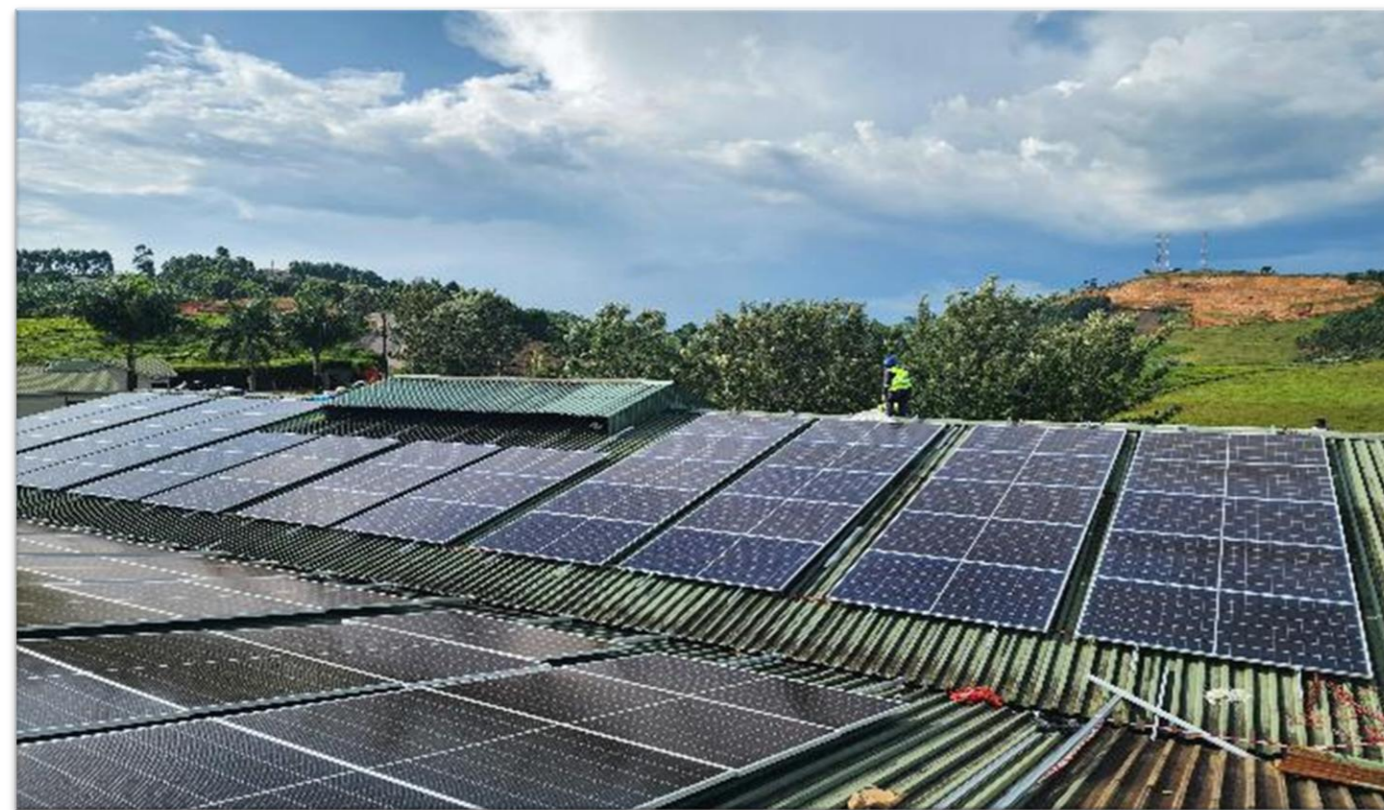
500 kWp Solar Panels 200 kWh battery back-up Kyamuhunga Tea Company , Bushenyi.
