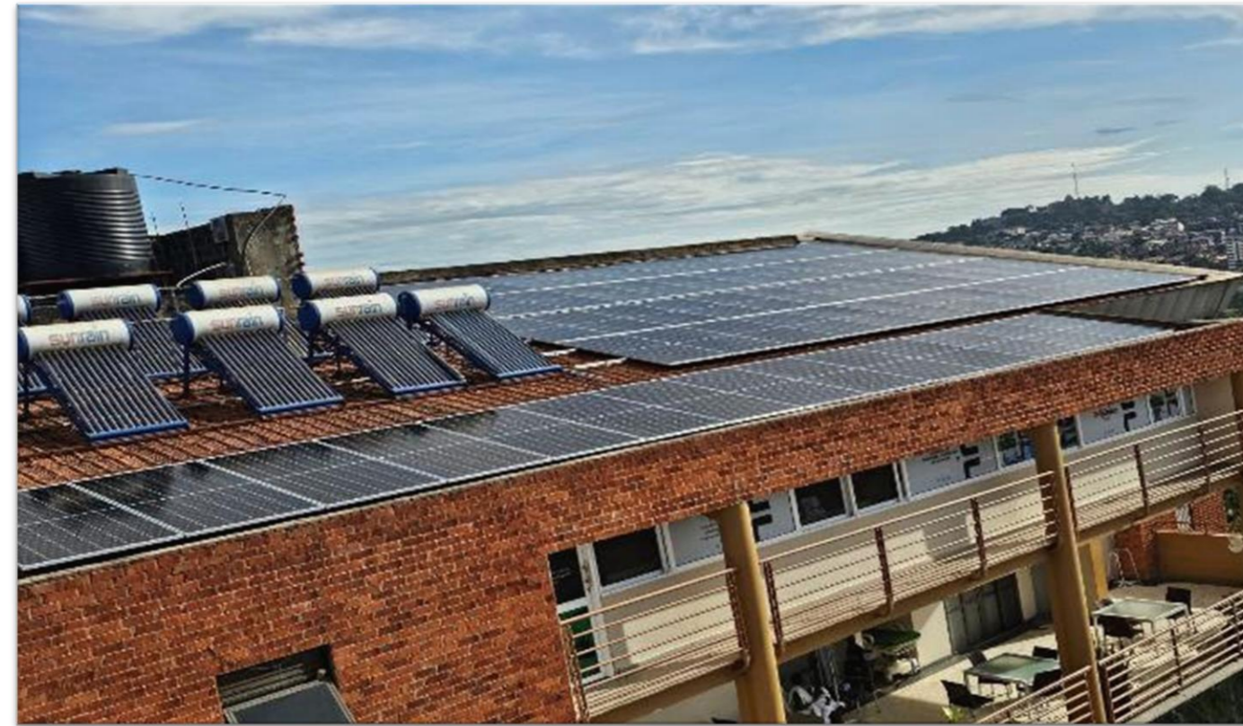
65 kWp grid tied system at Case Medical center , Kampala.
