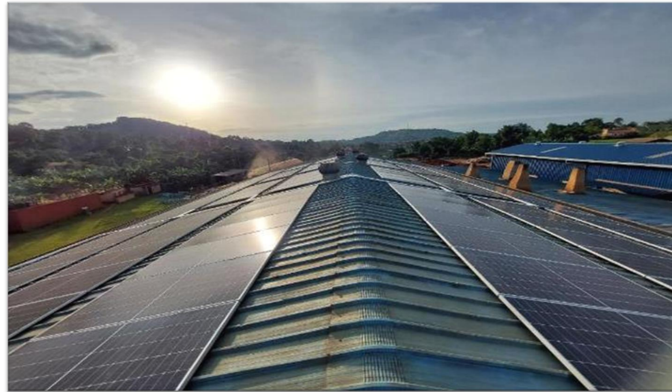
75 kWp Solar Panels 120 kWh Battery Back-Up Spouts of Water Factory , Kampala-Entebbe.
