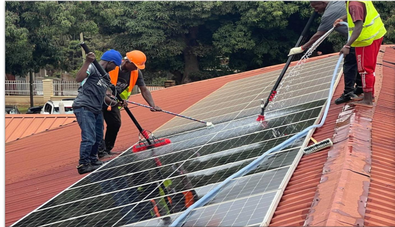
Corsu Hospital: Solar panel cleaning taking place.
