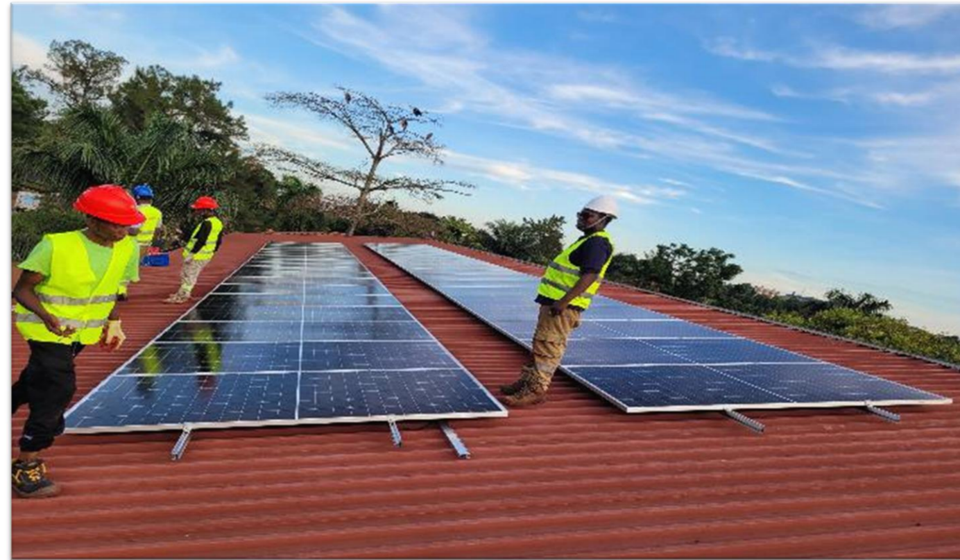
20kWp solar Pv solution for direct saving at Ambrosolis International School, Bugolobi.
