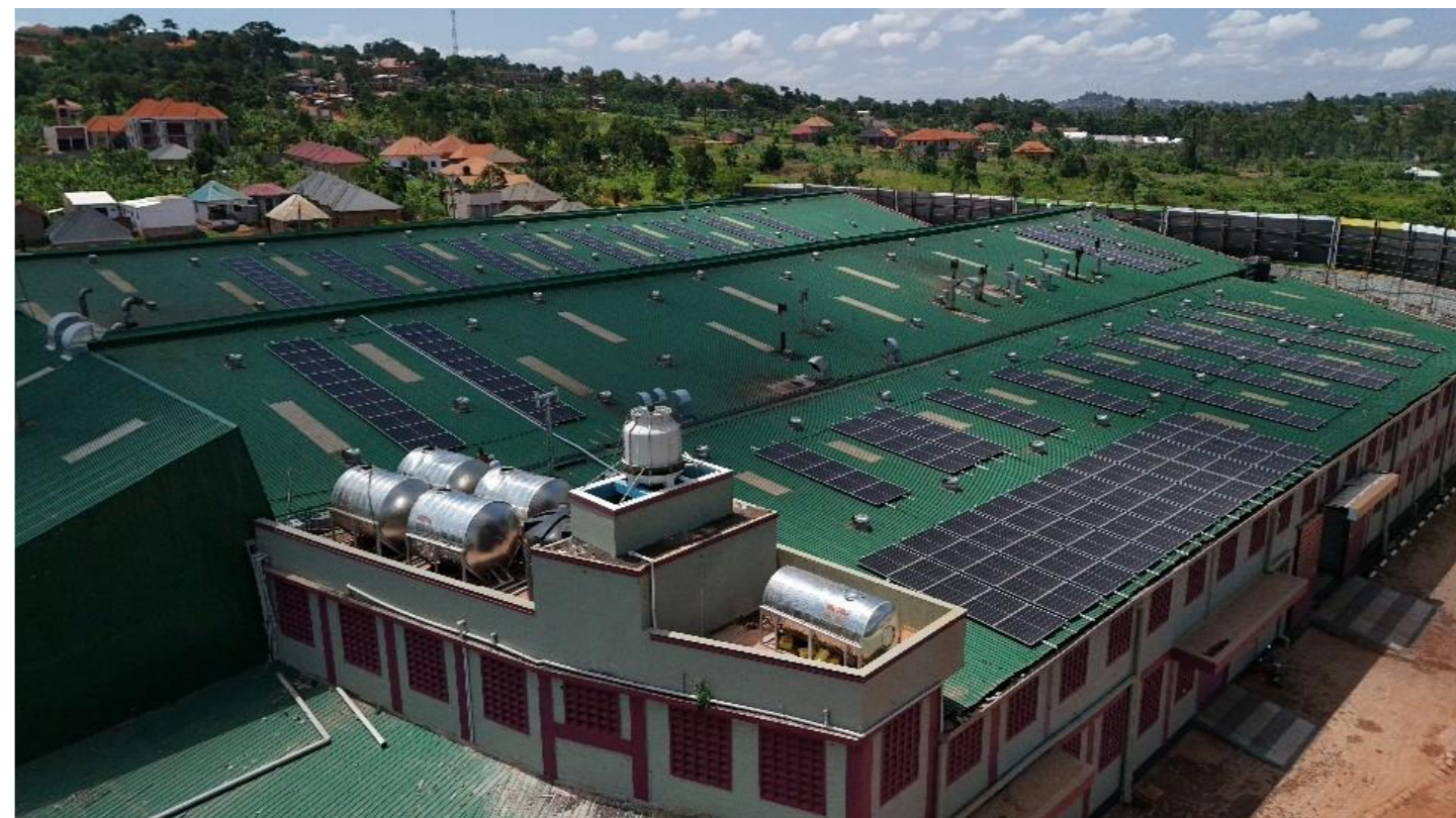
250 kWp solar panels grid connected at Psalms Foods Industries , Nansana..
