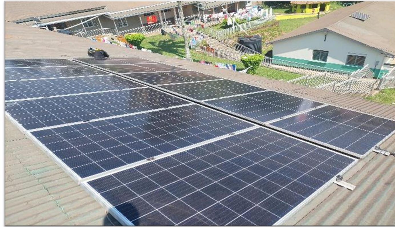
5kWp solar PV at Toro Babies home in Fort Portal Kabarole.
