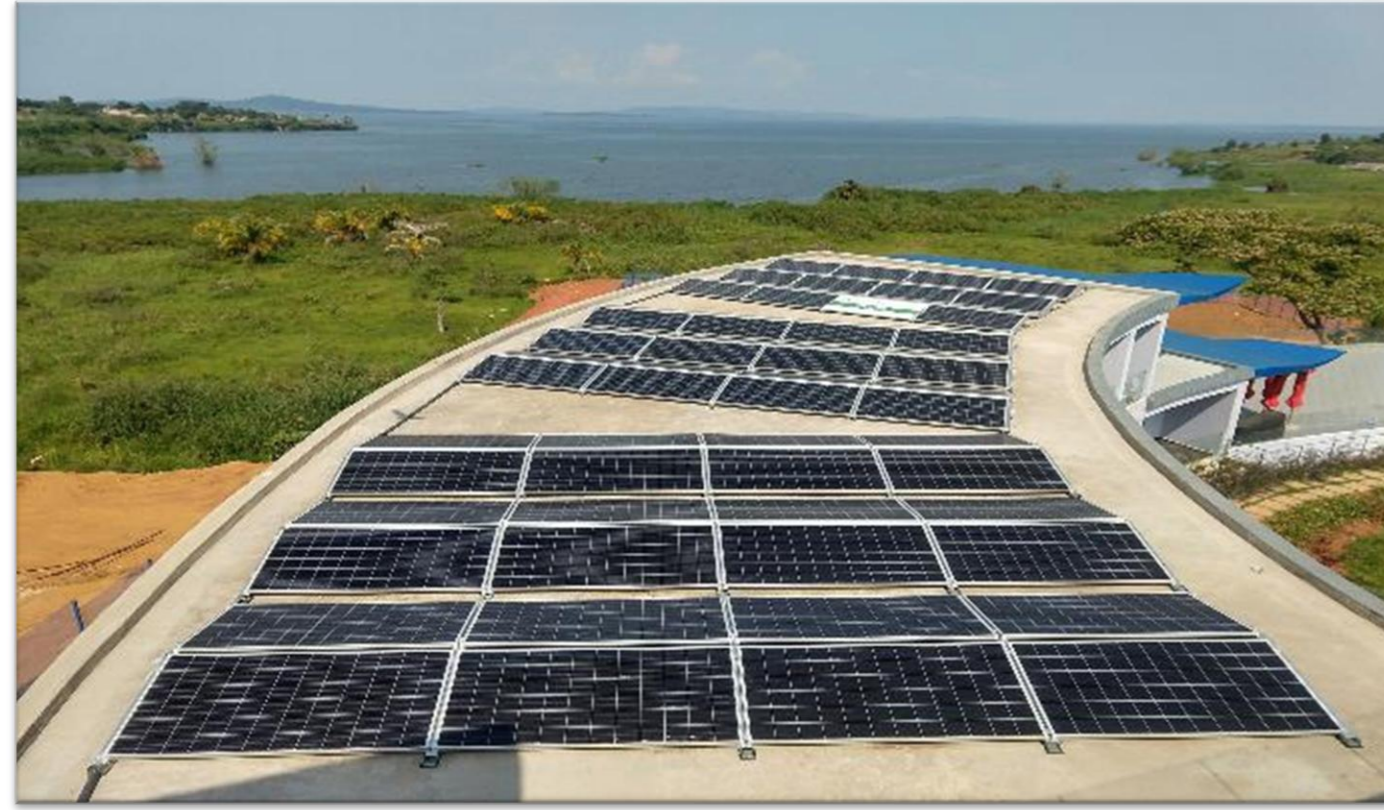
28 kWp solar system with grid connection at Aquarius Resort , Kigo.
