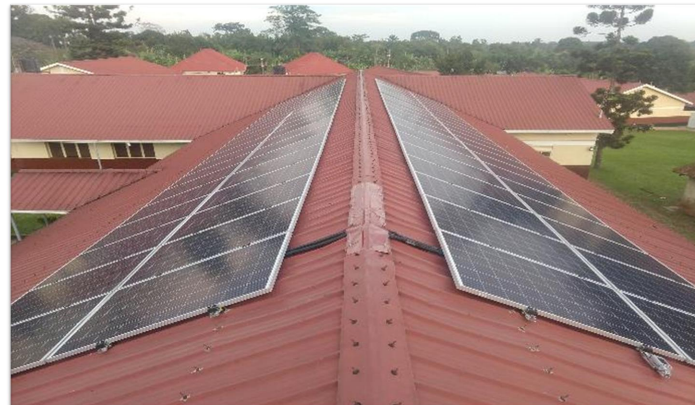
Solar PV System extension with 22 kWp of solar panels and 21 kWh at Nagalama Hospital , Nagalama.
