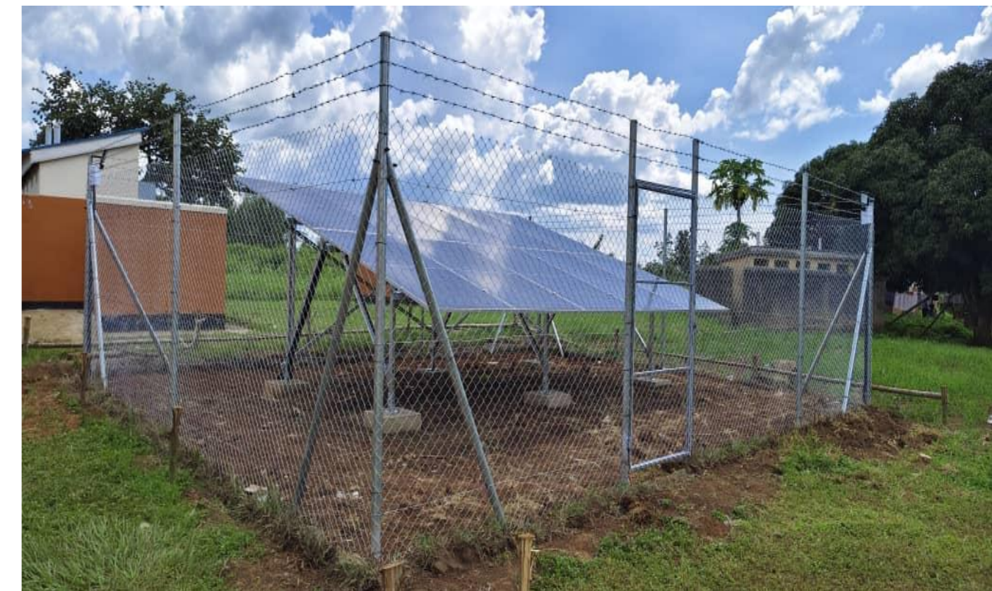
Installation of 3 to 10 kWp and 5 to 15 kWh PV Solar Systems at 250 Health Centers in Uganda , in cooperation with UNICEF and Ministry of Health Uganda .
