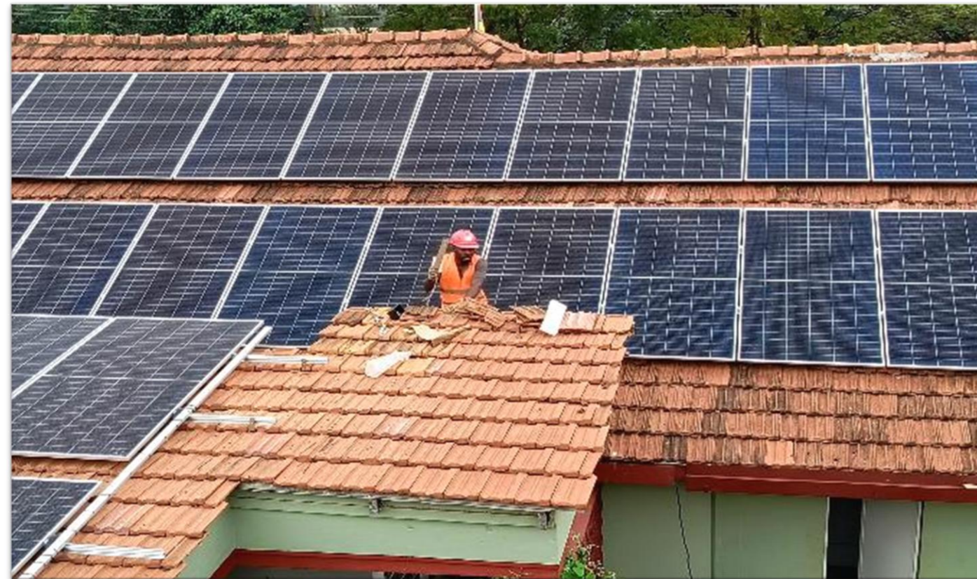
30 kWp solar system and 96 kWh battery back up at Masindi Hotel , Masindi.
