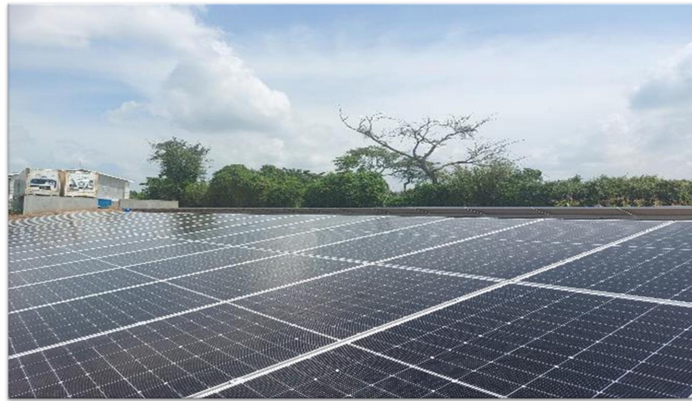
50 kWp solar panels Grid connected Misty Mountain Dairy Farm , Kapeeka.
