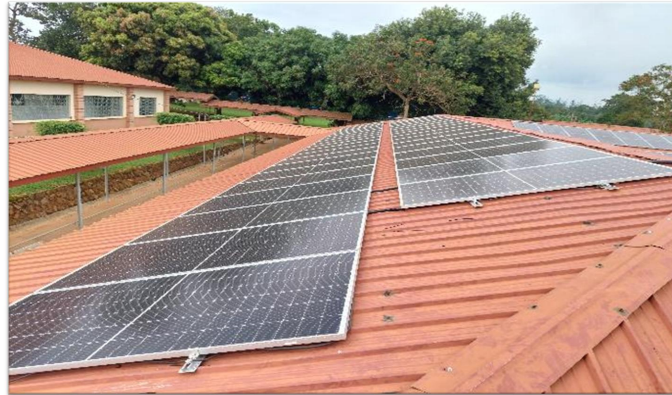
100 kWp Solar PV solution, 120 kWh solar back-up at Corsu Rehabilitation Hospital , Entebbe Kisubi.
