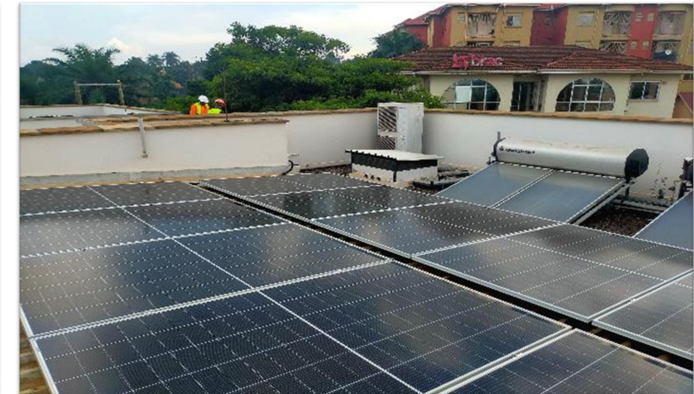
95 kWp solar system with grid connection at Quality Hill Mall , Gabba Road.
