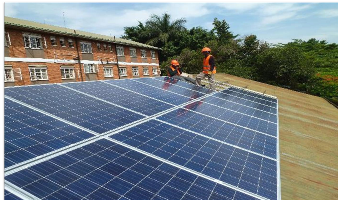
12 kWp at Uganda Catholic Management and Training Institute, Kampala.
