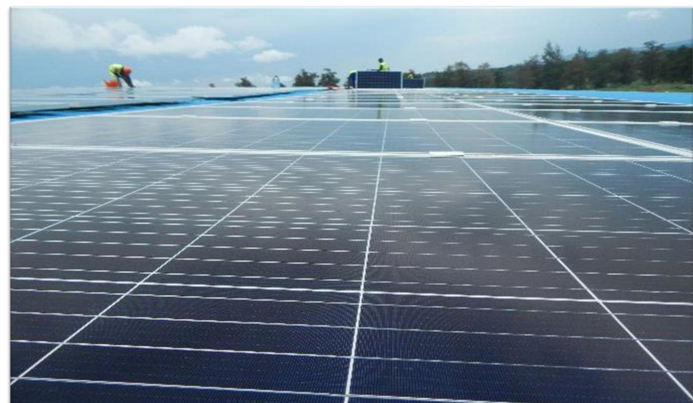
200 kWp Industrial solar PV solution at Jesa Farm Dairy , Busunju.
