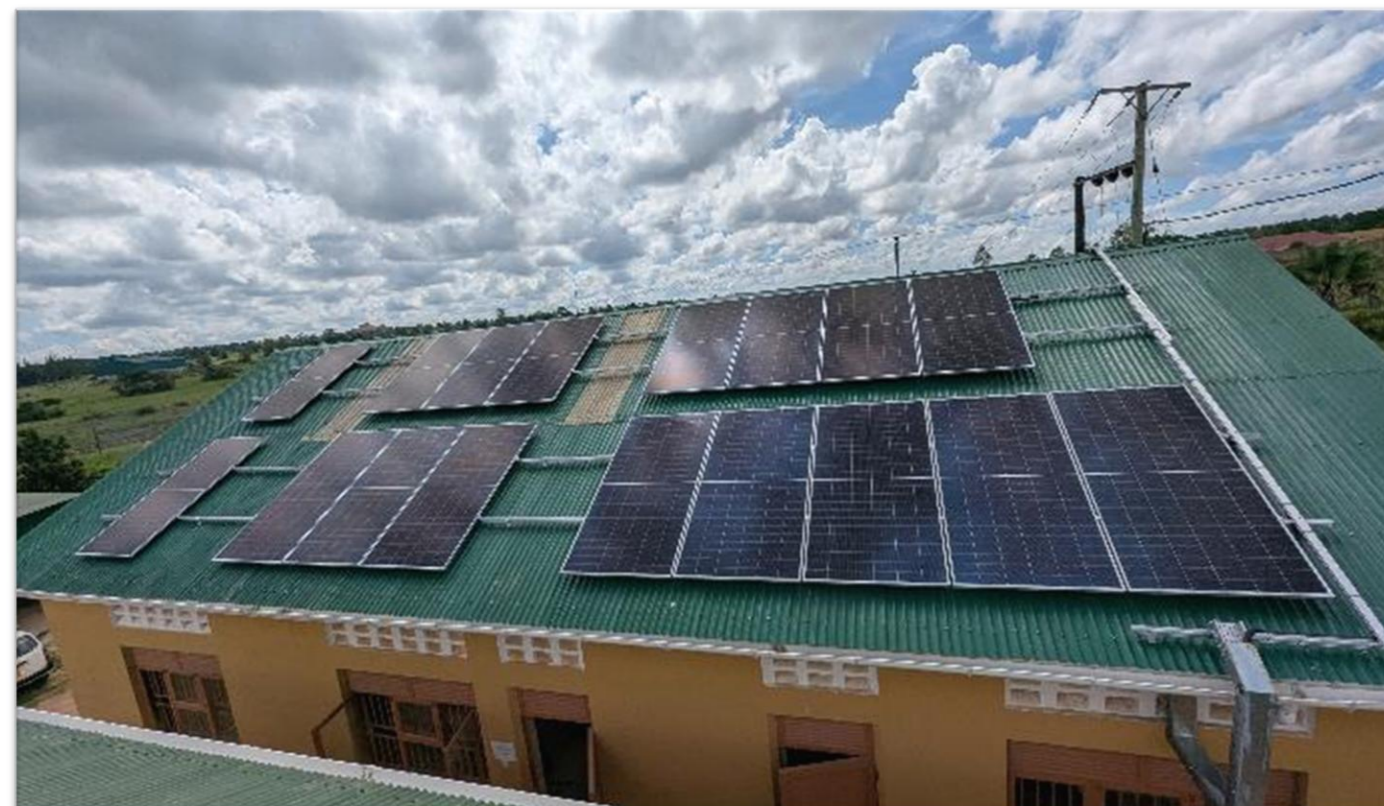
30 kWp solar PV solution and 30 kWh battery back-up at Soroti Youth Skills Centre Foundation, Soroti.
