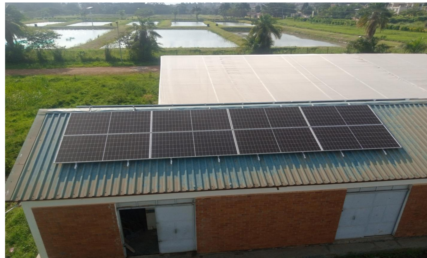
10 kWp solar pv solution, 9.6 kWh back up at Living Labs Kajjansi , Kajjansi.
