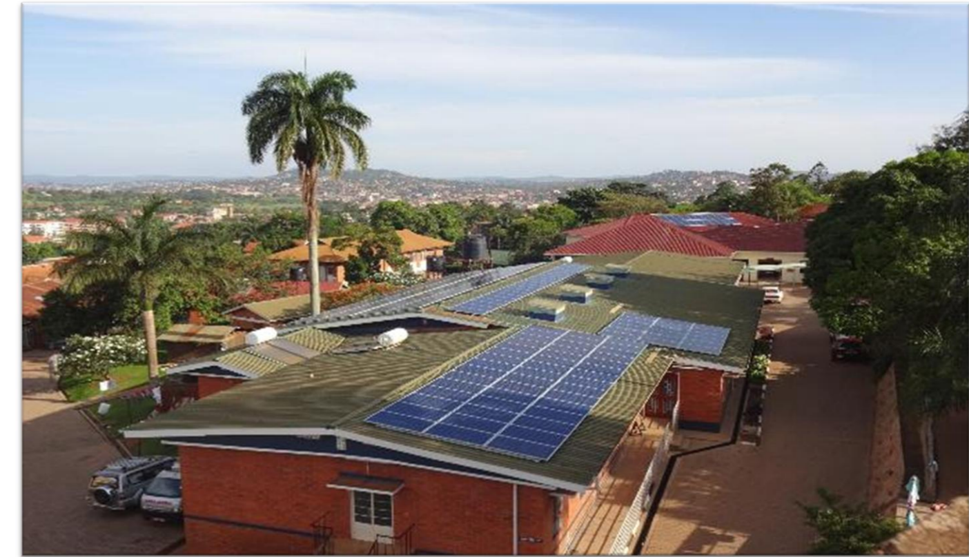
72 kWp Solar PV and Battery at Lubaga hospital Kampala.
